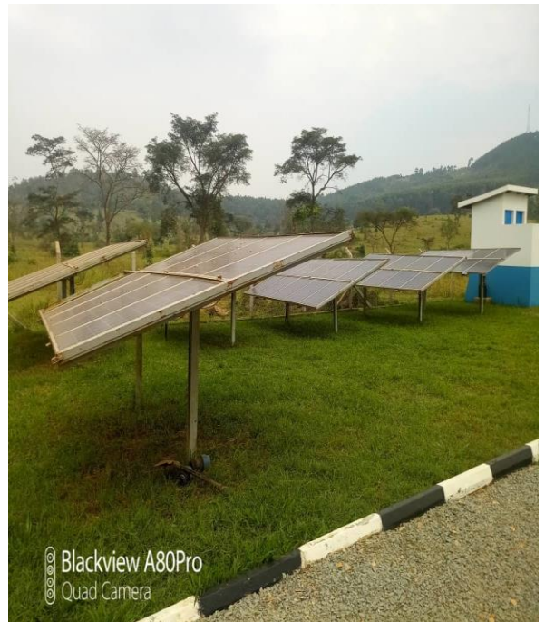
Figure 3: Solar PV array for Kashaka –Bubaare water scheme.
