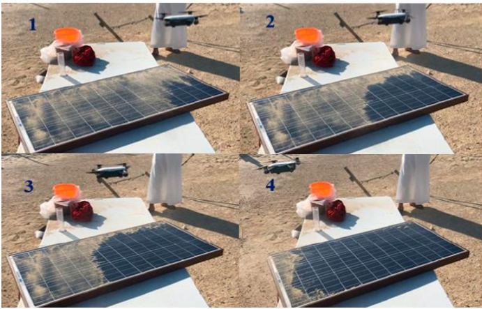
Figure 4: Dust accumulation in a Solar PV panel [27]
